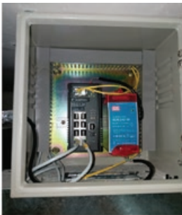
Multi-service Optical Network Units with 20Gbps uplink and full fiber redundancy with Fiber-to-Everywhere installation
